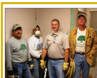
Camp Tyler Project - Robert Aiken, far right, and Kerry Hamblett (beside him) lead workers through renovations at Camp Tyler in December.
